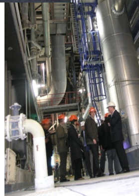
Castor Pilot Plant (2t/d)
